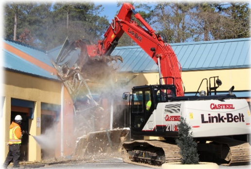
A backhoe tears down the top of the roof of the old Riverside Plaza
